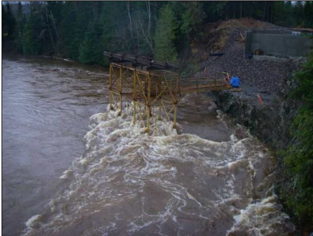
Figure 110. In late summer of 2008 contractors began to replace the Tabor Bridge. Photo shown of strong fall flooding taken following heavy rain events of late October 2008. Monitoring was conducted by HRAA staff and DENV to limit the impact of the construction on the river. Photo T. Benjamin.
