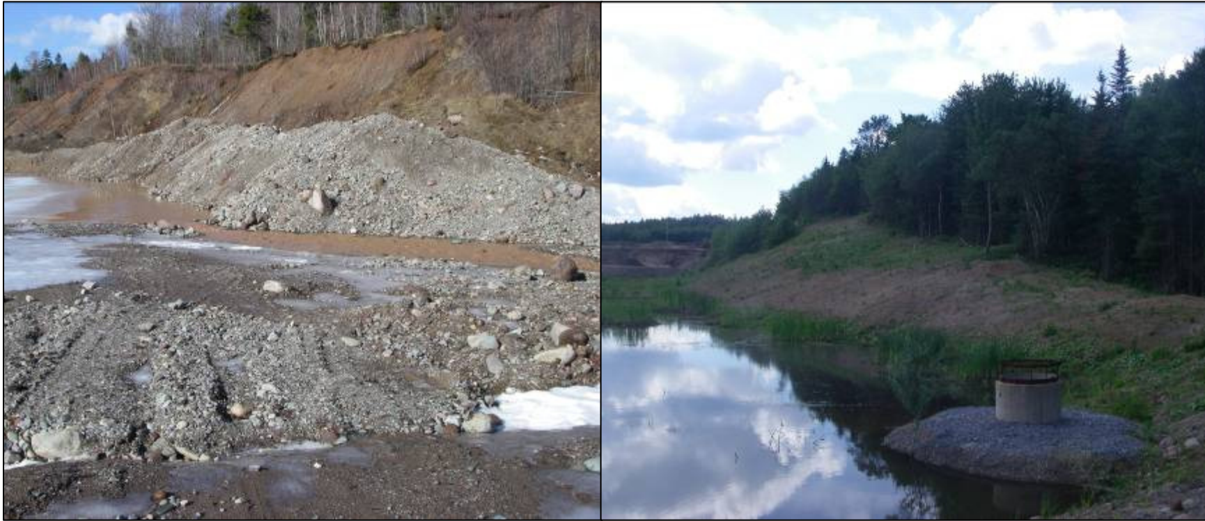
Figure 107. Renforth construction worked with HRAA staff and DENV to re-establish a degraded gravel pit reducing large flows of sediment to Palmer Brook. Photo on the left shows the Renforth pit in February of 2008 and the photo on the right show the same location in July 2008. A settling pond and standpipe was installed to regulate water runoff and prevent the sedimentation of Palmer Brook. Photos S. Campbell.
