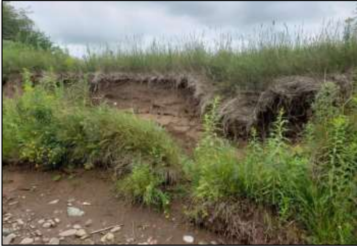
Figure 72. Sections of erosion along the riverbank near a hayfield.
