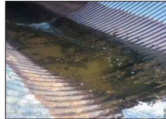
Figure 150. Degraded culvert of Desmond Brook. Photo: S. Blenis
