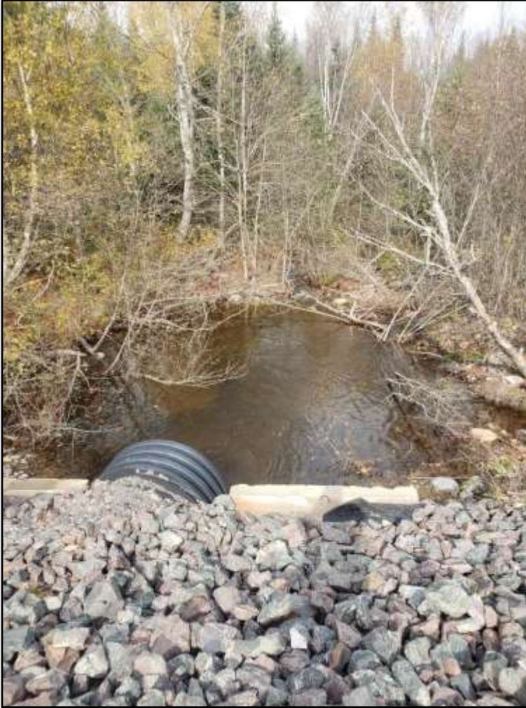
Figure 43. Looking downstream of Quigley Brook, and the relatively new culvert and the lovely, deep pool at the outflow. Photo: S. Blenis
