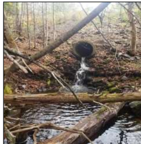
Figure 146. Hung culvert, with fairly deep outflow pool. Tributary should be assessed for fish presence, to determine priority of culvert replacement. Water Quality needs assessed in 2021. Photo: S. Blenis
