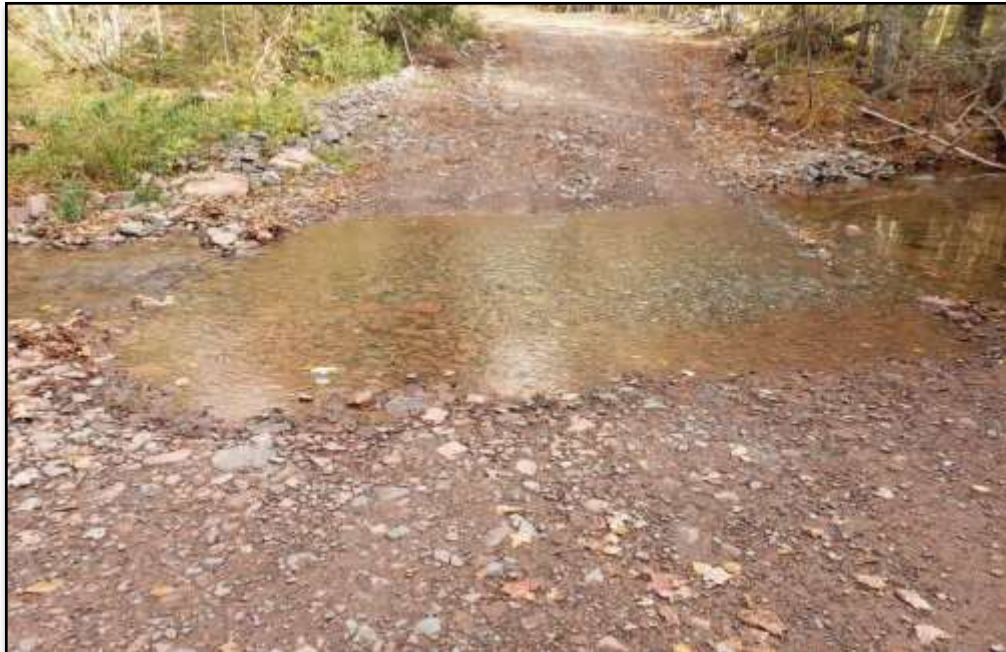
Figure 115. A dirt road crosses through the lower portion of Freddy's Falls tributary. A culvert or ford would assist in decreasing turbidity and sedimentation into the lower stretch of Freddy's Falls, and subsequently the Hammond River. Photo: S. Blenis
