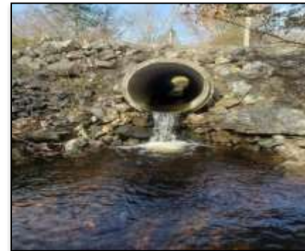
Figure 143. Severely hung culvert, does not allow fish passage, and poses a safety risk to motorists. Photo: S. Blenis
