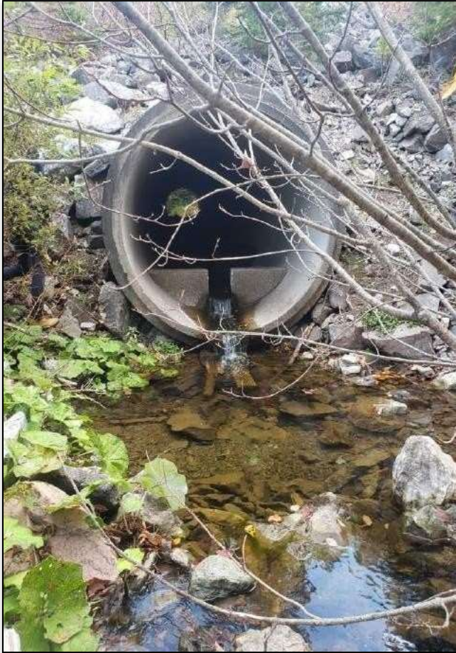
Figure 29. Baffled culvert in Markhamville, that baffled HRAA staff. Photo: S. Blenis
