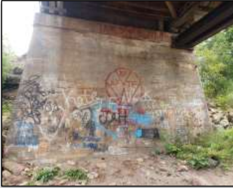
Figure 208 a. Graffiti covers the bridge pillar at Smithtown- a known hotspot for littering.
