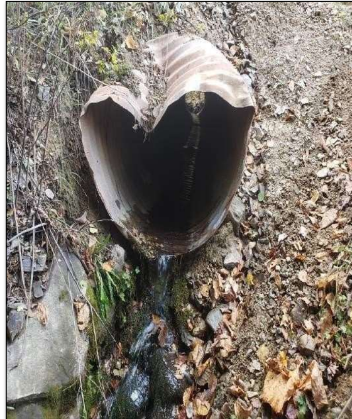
Figure 9. A deformed, poorly sloped, eroding, rusted culvert that does not allow fish passage, that was located on the Shepody Road in the Markhamville area on a dirt logging road. It's a real beauty! Photo: S. Blenis
