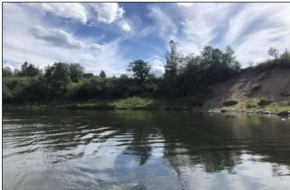
Looking upriver from Crowley's Pool, showing the proximity of the eroded bank to the road. Photo: J. Kelly
