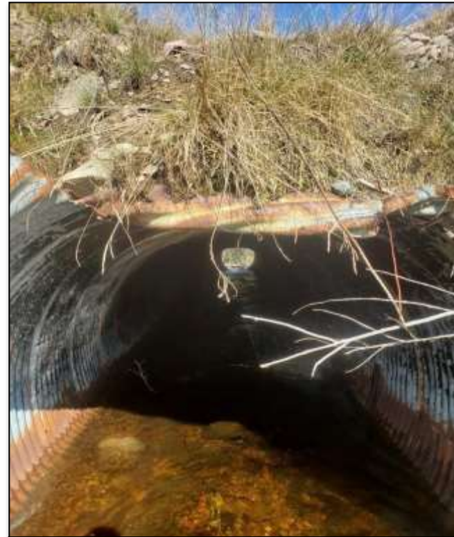
Figure 82 . An extremely compromised culvert under route 111 and connects the beaver area of Isaac Brook to the main outflow of the brook. The bottom of the culvert has completely rusted out, and the culvert has become compacted, with severe erosion issues on the crown. This culvert receives a high priority ranking for repair, as it possesses a future safety concern for traffic. Photo: S. Blenis
